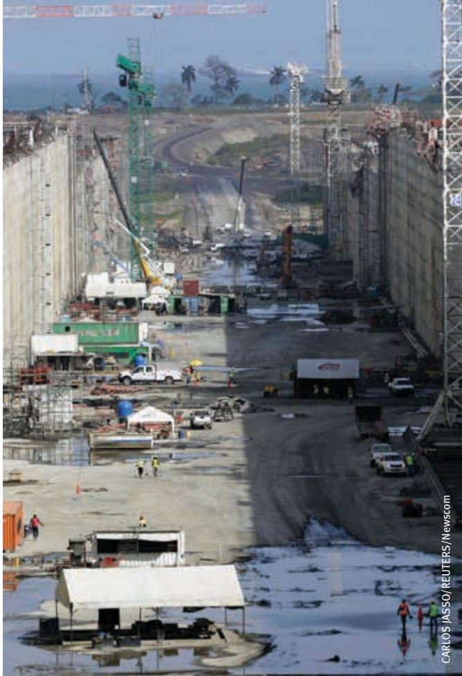
Workers and cranes are seen at the construction site of the Panama Canal expansion project on the Atlantic side on the outskirts of Colon City on January 15, 2014.
